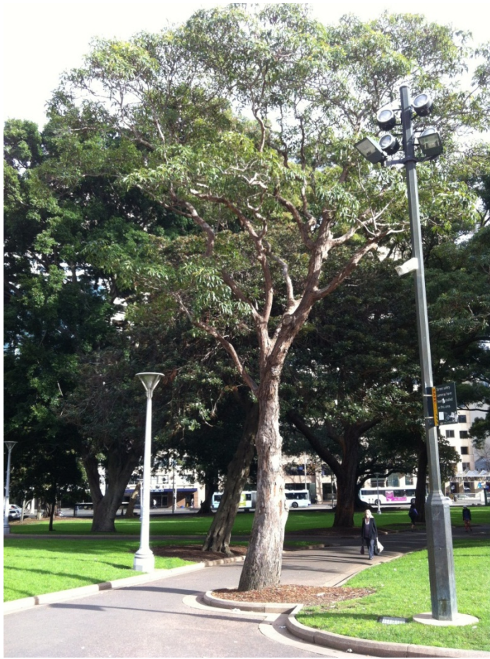
Tree 360S Brush Box (west of Pool of Reflection). Reason for removal - previous construction root damage, and the tree is in decline.
